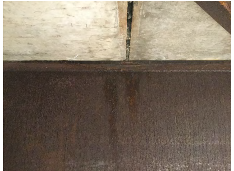
Right span water getting through deck joints
