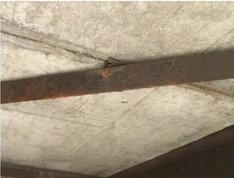
Right span corrosion on bracing
