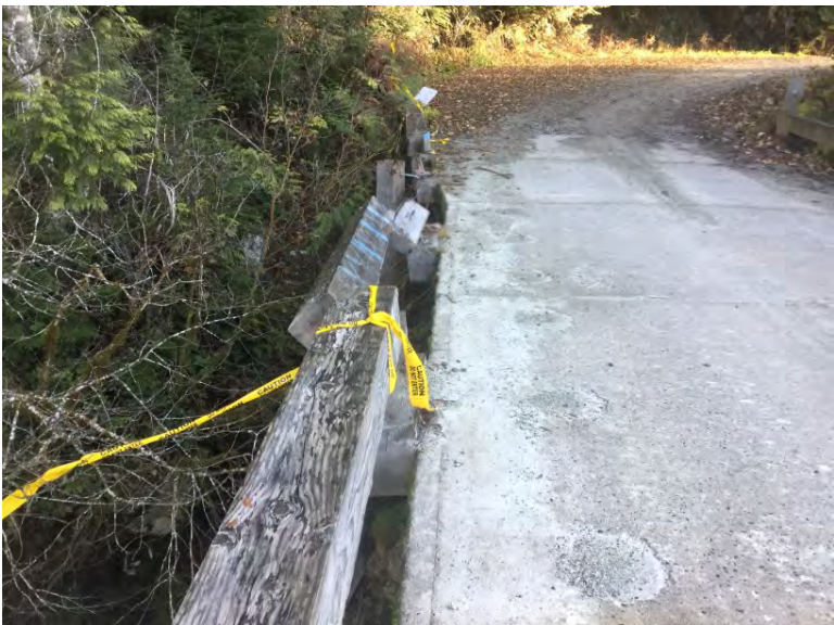
Guardrail damage at upstream left approach
