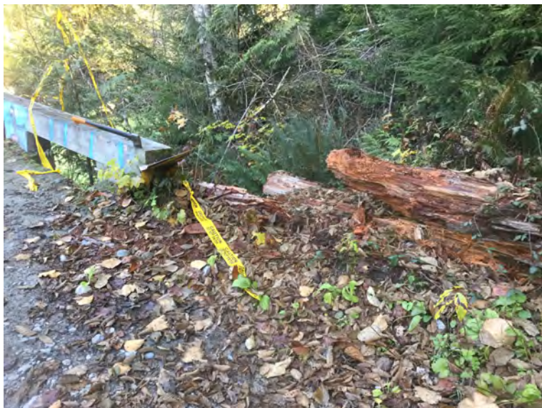
Upstream left approach fender condition
